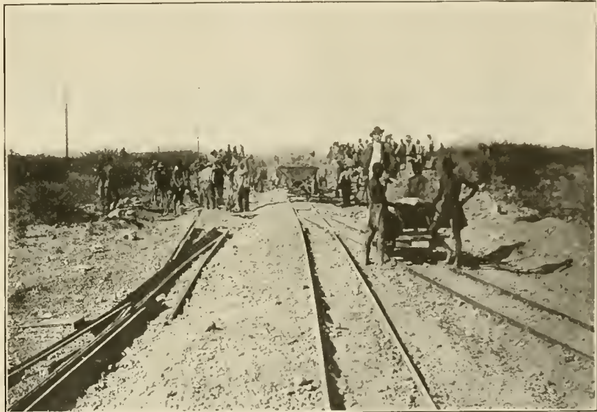
NATIVES AT WORK ON THE PERMANENT WAY OF THE OTAVI RAILWAY. SOUTH-WEST AFRICA.
